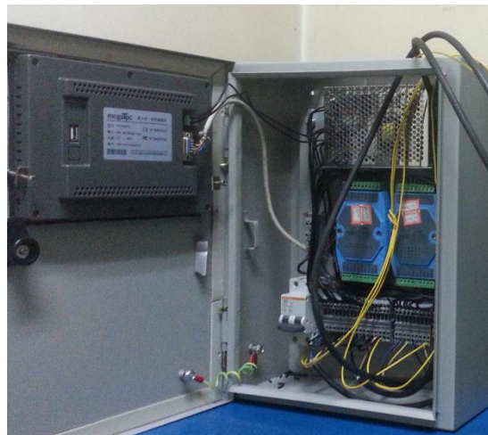
Figure 6 New signal conversion box in debugging process
